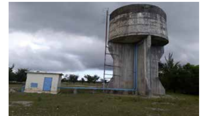
Plate 4. 1: The water storage tank for the Kiuyu-Mbuyuni and MaziwaNg'ombe scheme
