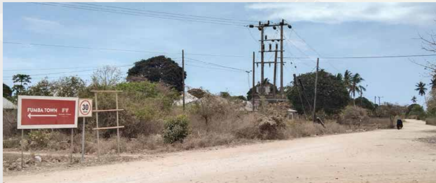
Plate 5. 9: Existing 33kv Transmission line at Nyamanzi with 100KVA transformer energized
