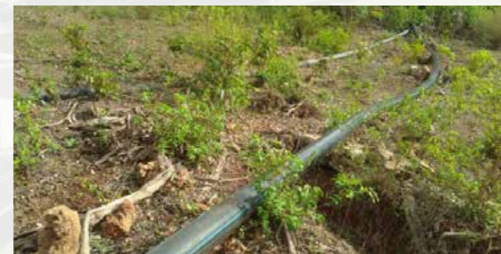
Plate 5. 4: Water main and appurtenances from Dimani sources to Fumba area
