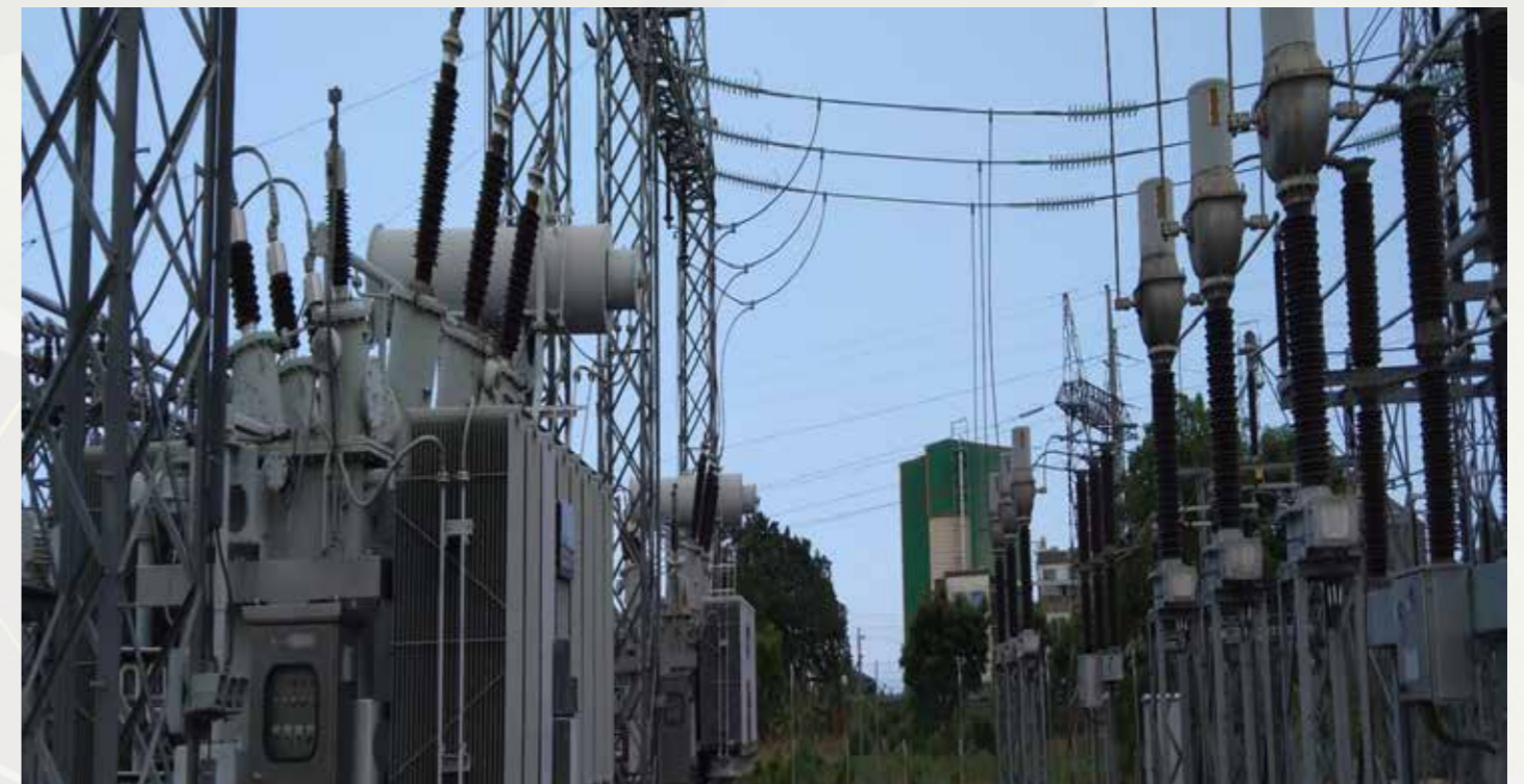
Plate 5. 10: New 100MW,132KV substation with total electric power consumption minimum 50MW to Maximum 85MW.
