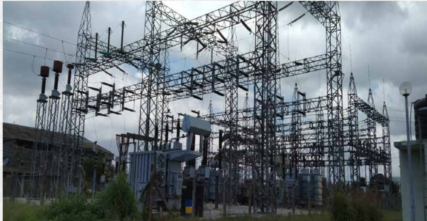
Plate 5. 8: Old 45MW,132KV substation
