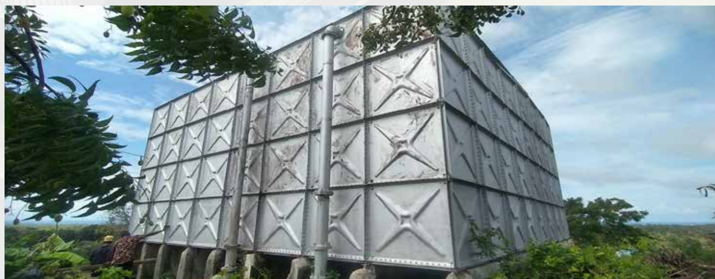
Plate 5. 3: The storage tank of 300,000 litres located in Dimani
