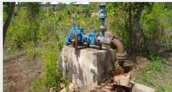
Plate 5. 2: Borehole which yields of 60m 3 /h
